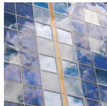
➤ Building integrated photovoltaic (BIPV)
